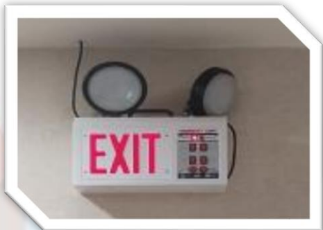
Battery Operated Emergency lights in Corridors/stairs
