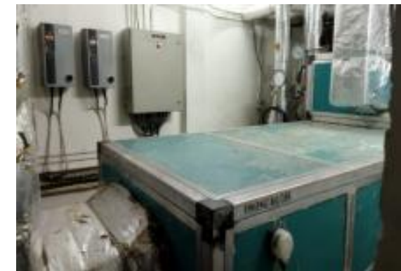
AHU with VFD
