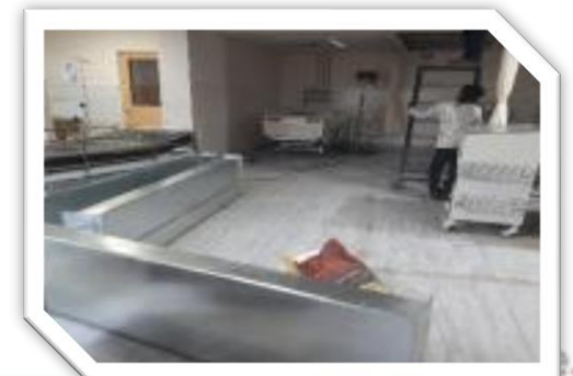
Modification in ducts for Two OT's ran with one AHU
