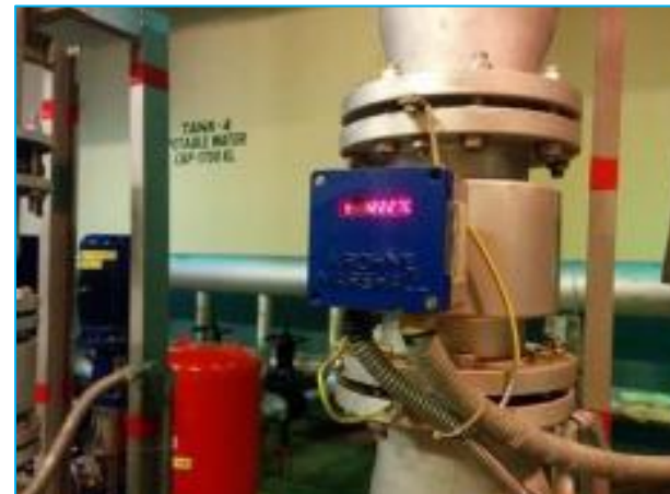
System level Water Metering facility
