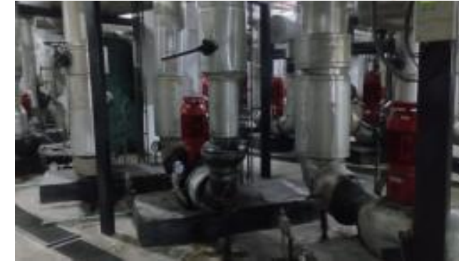
HVAC Primary Pump Stoppage
